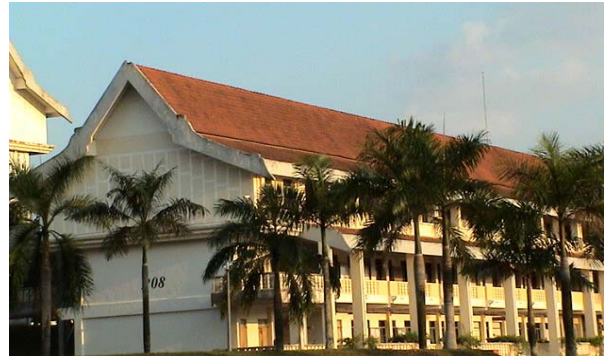
Fig. 2. The same building was also struck and damaged by lightning at the northern ridge end. The silhouette of the ESE system can be seen on the roof at right about 20m away.
