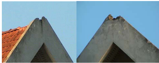
Fig. 3. Close-up photographs of the lightning damaged ridge ends.
