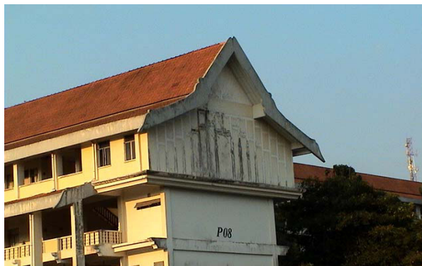
Fig. 1. The UTM electrical engineering building (Block P08) that was struck and damaged by lightning at the southern ridge end.
